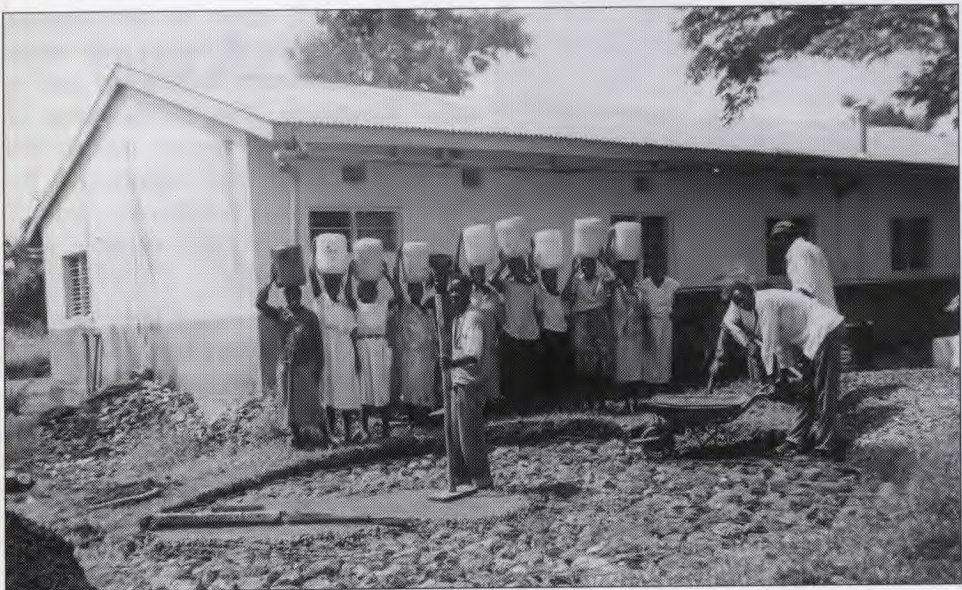
The women bringing water for the river to make concrete. This went on for five days!
