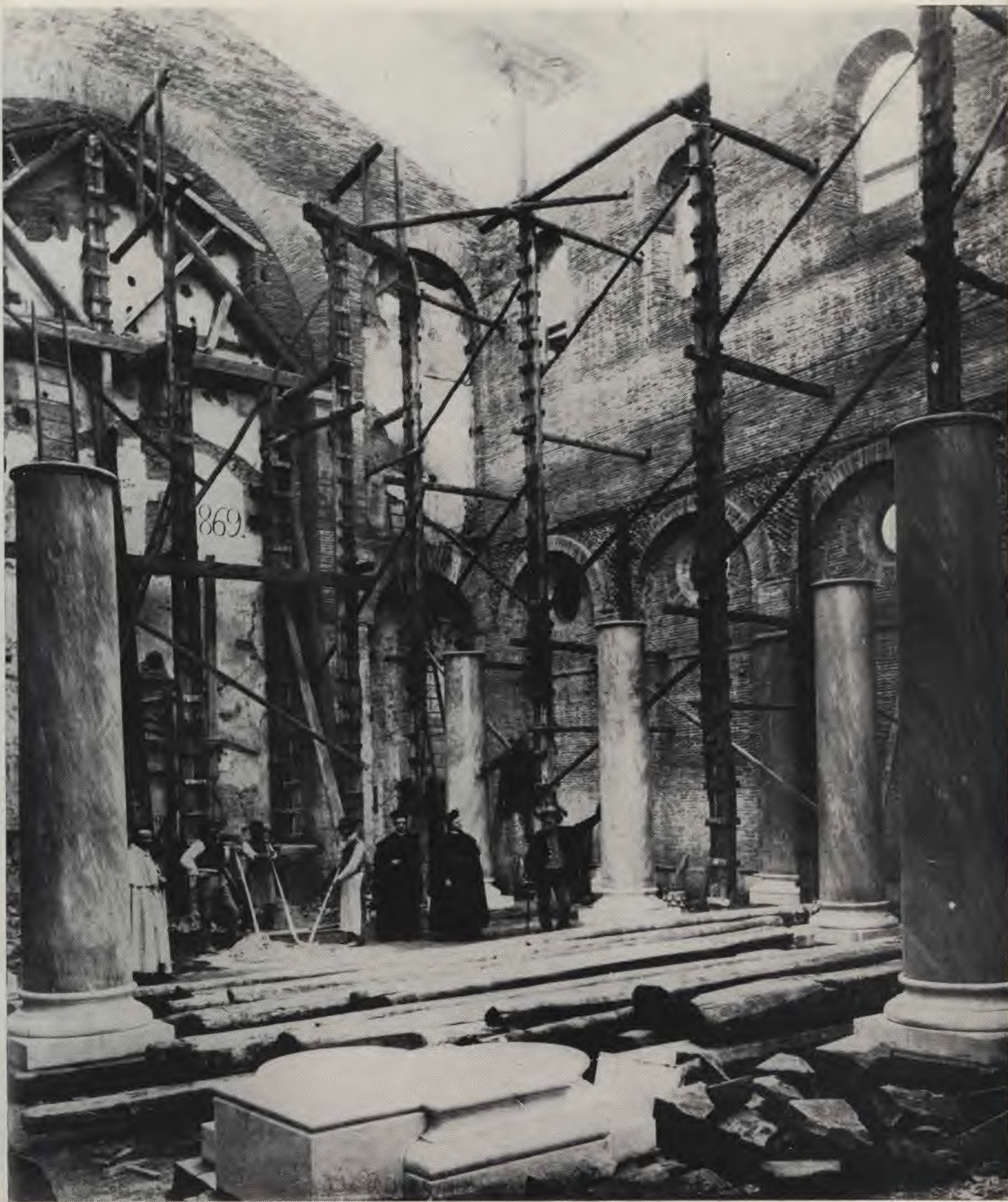
The College Church under construction, 1869. Surveying the work are Mgr Henry O'Callaghan (left), Rector 1867-88, and Mgr George Talbot, Pro-Protector of the College
